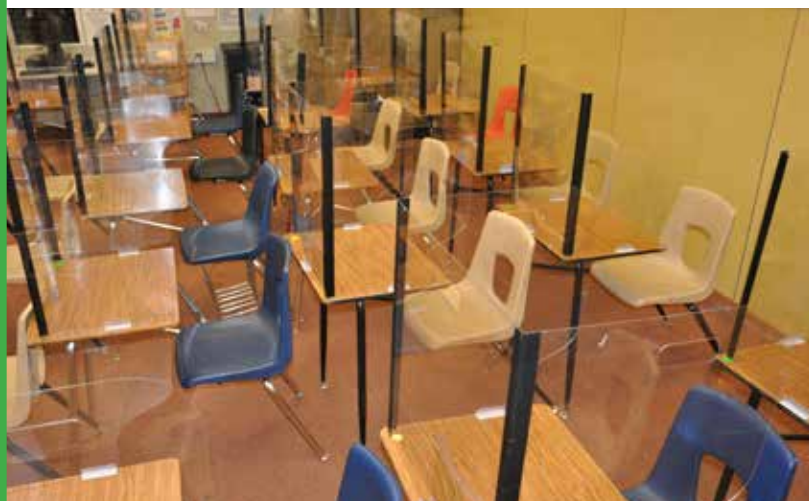
Every desk, in every classroom, needed to be fitted with plexiglass barriers.
